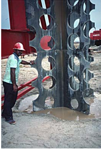
Fig. 13. Liquefaction of water-saturated sand during the initial phase of compaction. Note that the ground water level is 4.5 m below the ground surface.
